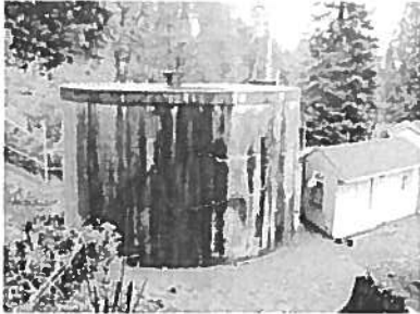
Grandview Terrace reservoir
