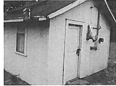
Hillside pump station
